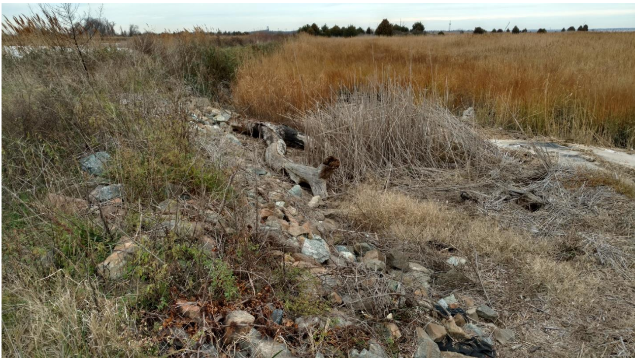
Figure 20. View to north showing Stone mantling (riprap) along river face north of the sluice. Embankment to left of image.
