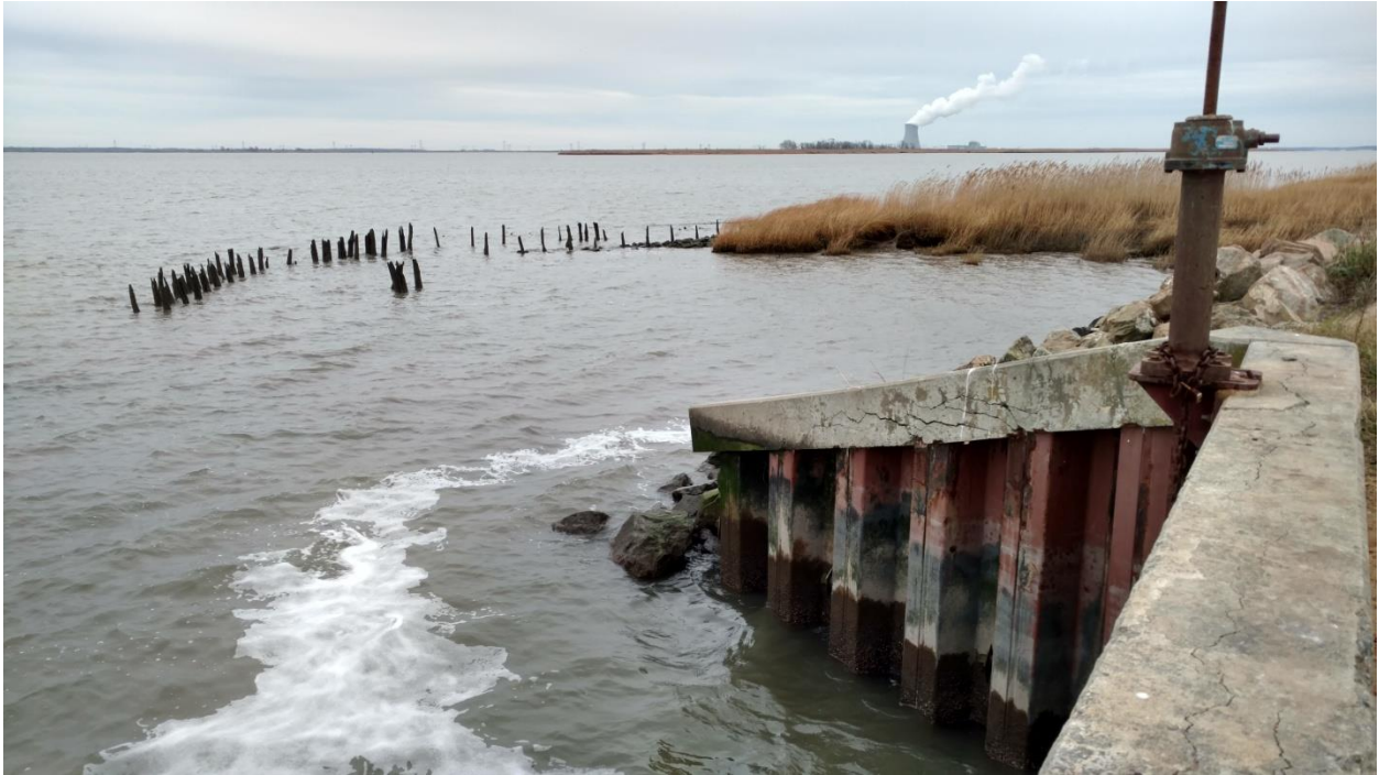
Figure 26. View to the east looking at the timber configuration south of the sluice entrance.
