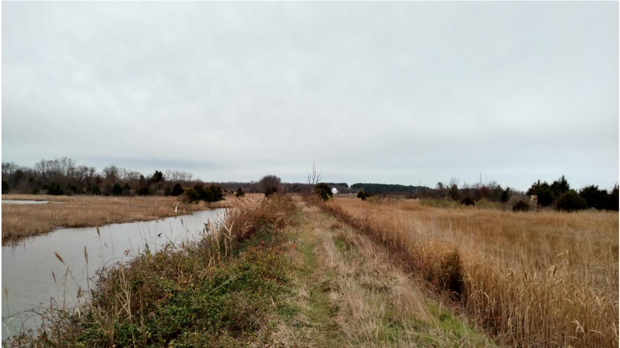
Figure 17. View to the west along the northern embankment wall. Impoundment area to left of image.
