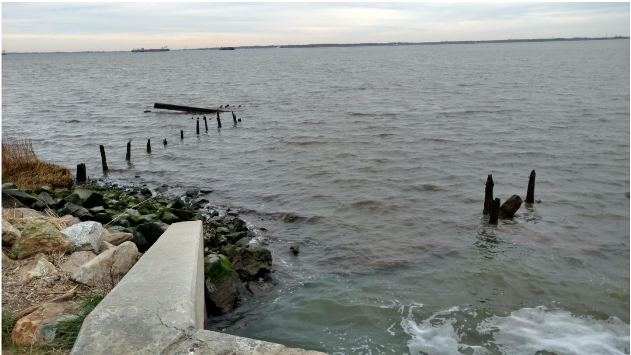
Figure 27. View to the east toward the river, showing the timber configuration north of the sluice.
