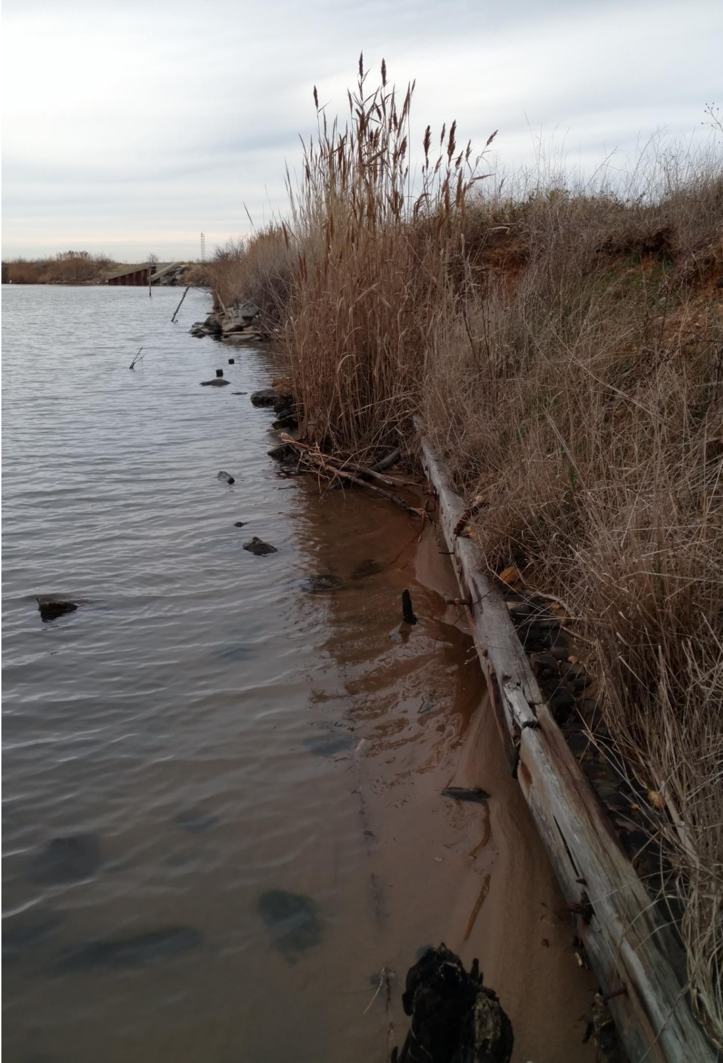
Figure 23. View to the northeast of wooden cribbing on the interior of the southern embankment.
