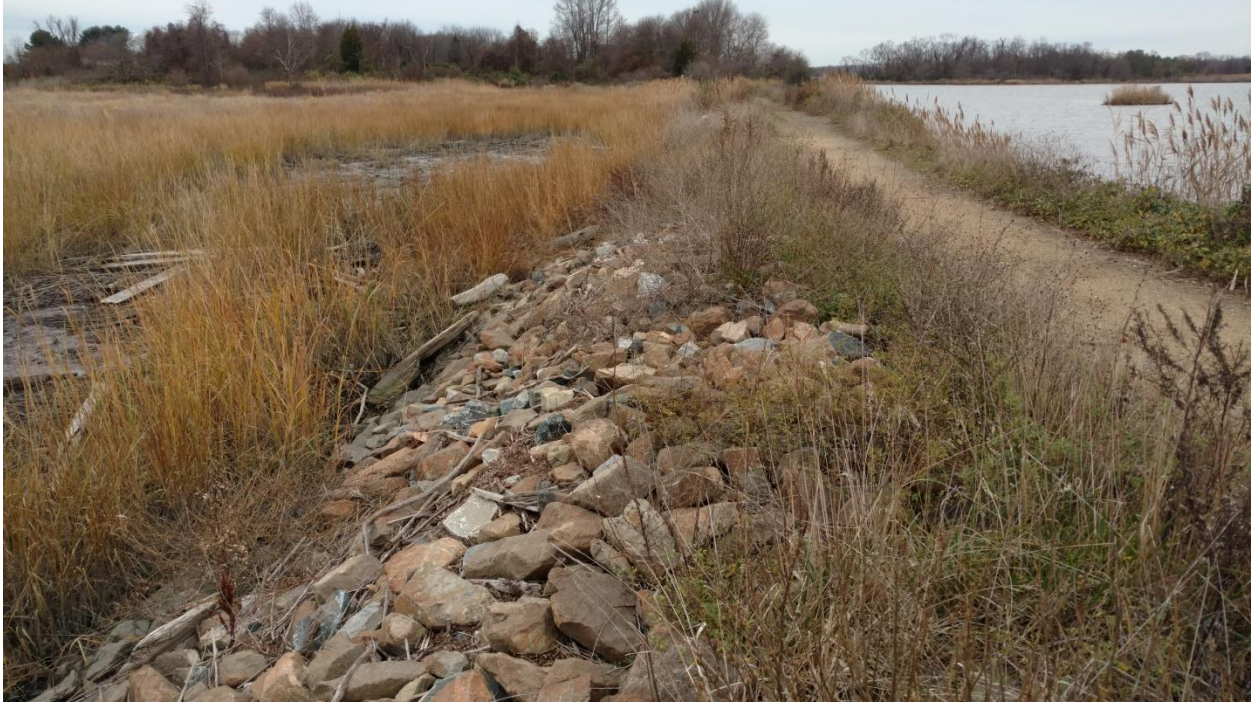
Figure 24. View to the southwest showing the southern embankment and stone riprap along the exterior (river side) of the embankment. Impoundment to the right, and the Lang Headquarters area is in the trees in the center distance.
