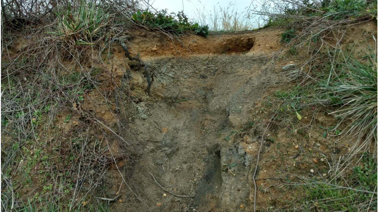
Figure 21. View to east of exposed section of the earthen dike, showing clay core and sandy overmantle. This section is south of the sluice.
