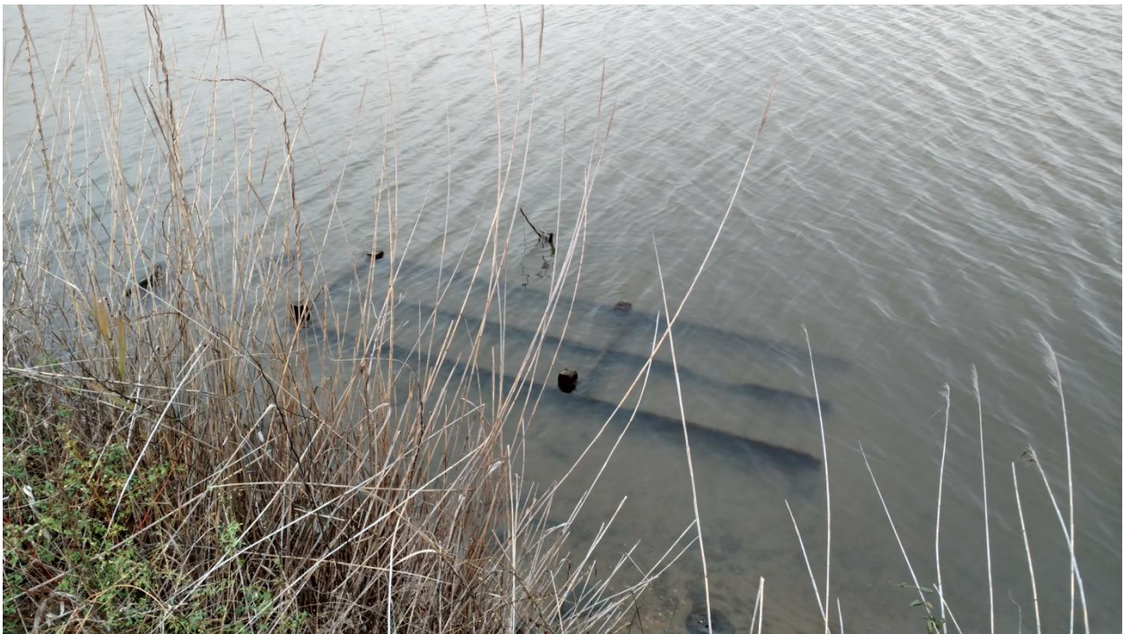
Figure 22. View to the interior of the impoundment showing submerged cribbing. This is located along the southern embankment, south of the sluice.
