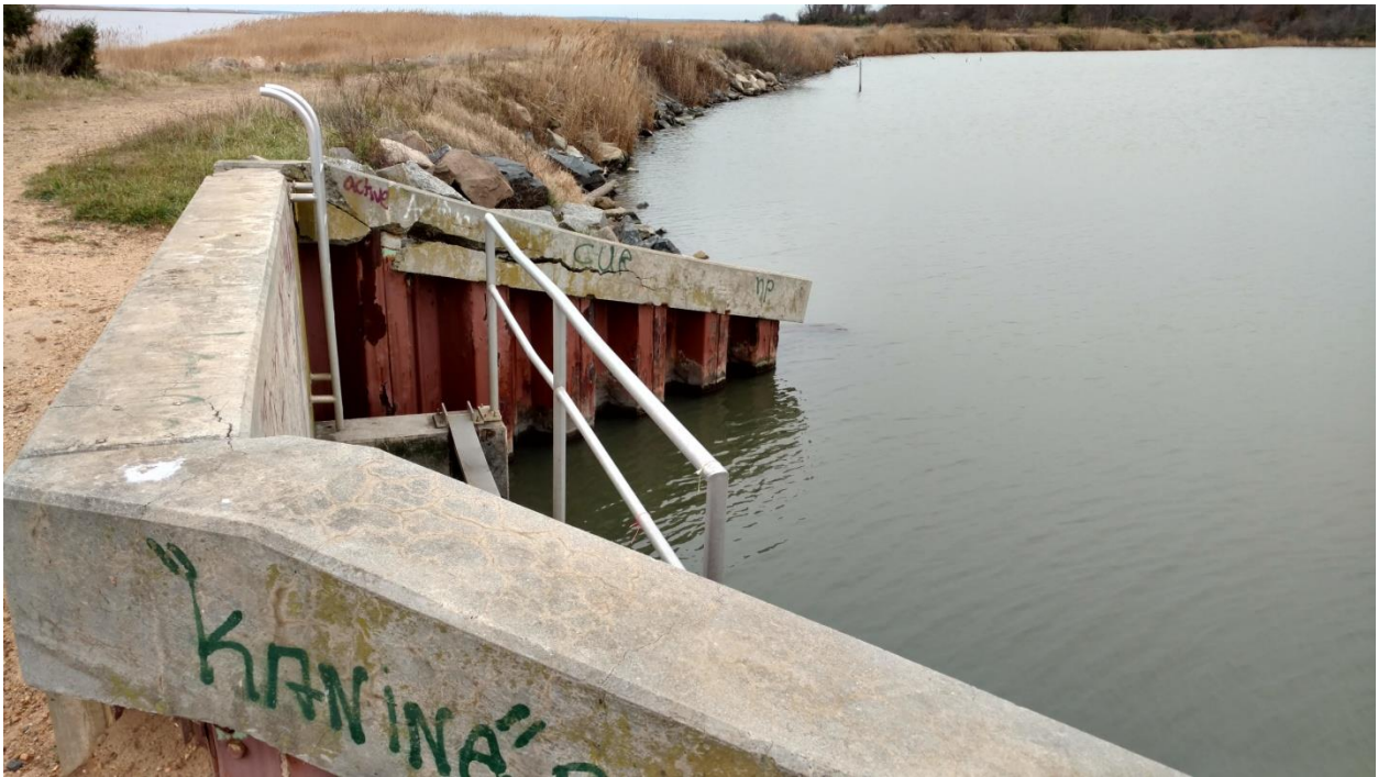
Figure 25. View to the south of the concrete and steel sluice. River is to the left, impoundment to the right.
